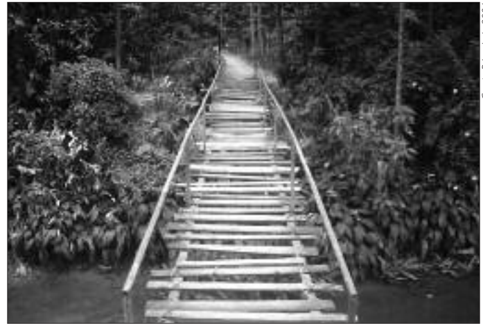
Weak, uneven water crossings can be hazardous (Sri Lanka)
