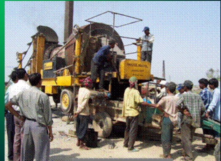
Hot Mix Plant
